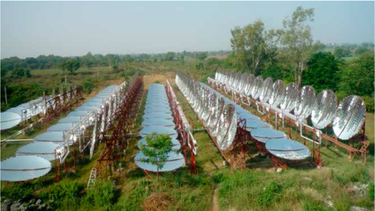
Parabolic solar collectors power the air conditioning system at Muni Seva Ashram Hospital in Goraj, India. (Photo: Urvish Dave's Blog & Muni Seva Ashram – Goraj)
