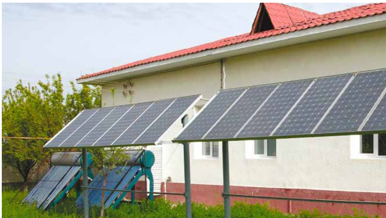
Solar-powered health centre in rural Uzbekistan. A recent government initiative aims to improve health services by harnessing solar energy as a source of reliable power and heating. (Photo: UNDP/Uzbekistan)
